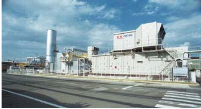
The Kawasaki L20A turbine has begun the commissioning process at Kawasaki's Akashi works in Japan
